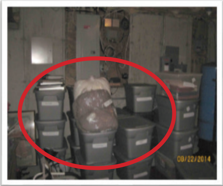
Photo D3: Working clearance not maintained: NEC 110.26
