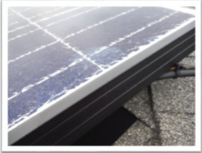
Photo D4: Equipment visibly damaged
