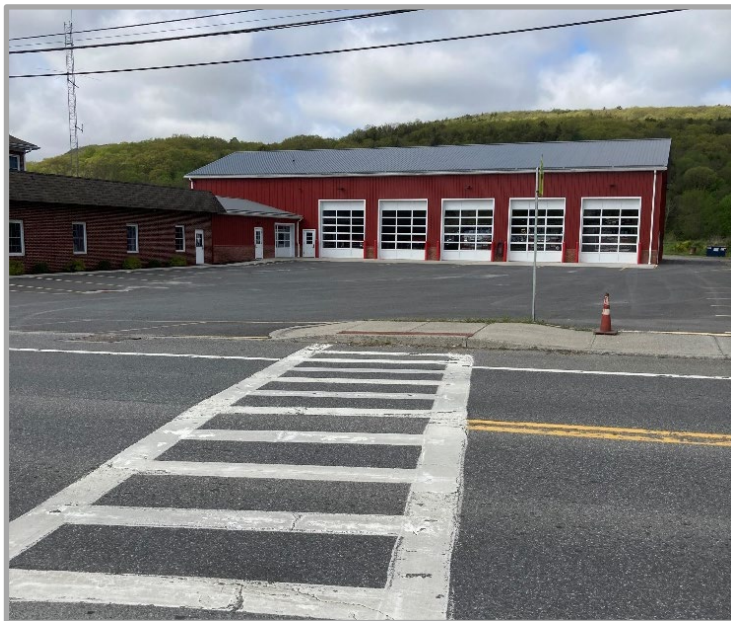
The Route 22 crosswalk at School St lacks a ramp on the west side.
