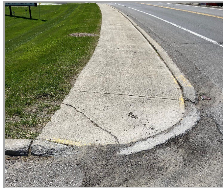
A curb ramp on Route 22 with no detectable warning.
